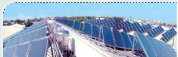
FIGURE 3: Stainless steel tanks have optimal hygienic properties (Photo: jj-solar.com )
