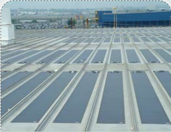
FIGURE 28: Flat stainless steel roof with integrated amorphous PV cells (Photo: uni-solar.com)
