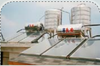
FIGURE 4: Long-term experience in rooftop applications is available all over the world. (Photo: jj-solar.com)
