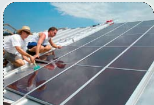
FIGURE 35: The trays of the stainless steel roof support the photovoltaic panels (Photo: protectum.de)
