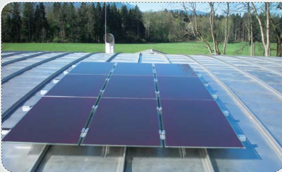
FIGURE 36: In flat parts of the roof, where rainwater does not flow off easily, the stainless steel welded seam option is the only possible metallic solution. (Photo: protectum.de)
